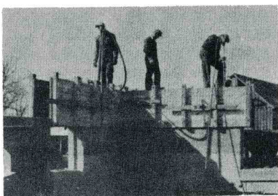
Pneumatic ramming of soil-cement walls in wood shuttering. Cameron Valley Project, Virginia
