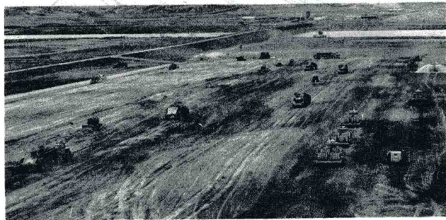
Hauling and sheepsfoot rolling for a section of Garrison Dam, North Dakota. Water sprinkler and disc harrows at right maintain proper moisture content for compaction.
