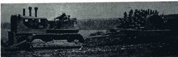
Sheepsfoot roller giving Oahe Dam (᠓·᠔·᠒᠒) its most vital ingredient, compactness. Compaction increases strength and decreases permeability. Check tests tell if soil densities meet specifications; if not, more rolling.
