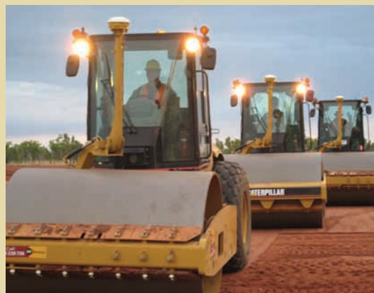
Researchers used GPS machine control, roller-integrated compaction monitoring, and rapid soil stabilization technologies to create an unsurfaced runway.
